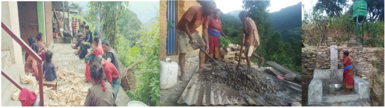
Picture 1: Water Wastage (lack of storage). Picture 2: Temporary arrangements for intake of water. Picture 3: Tap conditions Picture 4: Meeting for new water scheme Picture 4: Sand Cement Work for Construction 6: Construction of New tap.
