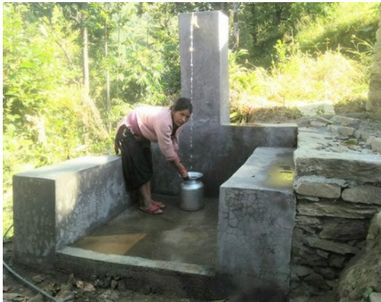
Picture 1-2: Transportation of plastic drum. Picture 3 -4: Construction of tap. Picture 5: Local making use of tap to collect drinking water.
